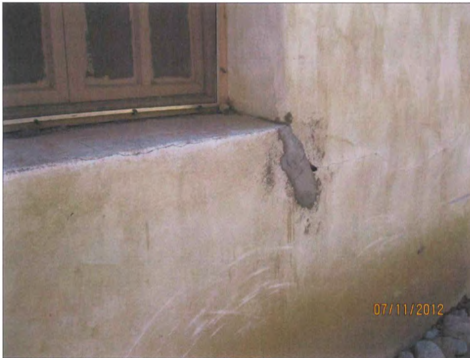
Photo illustrating general “wear-and-tear” to be repaired
