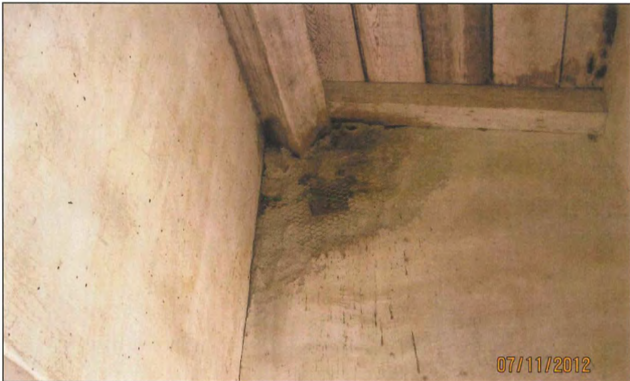
Water-damaged cement – based plaster installed during late 1940s restoration to be removed and replaced with a lime-based plaster (for improved breathability) on an as-needed basis
