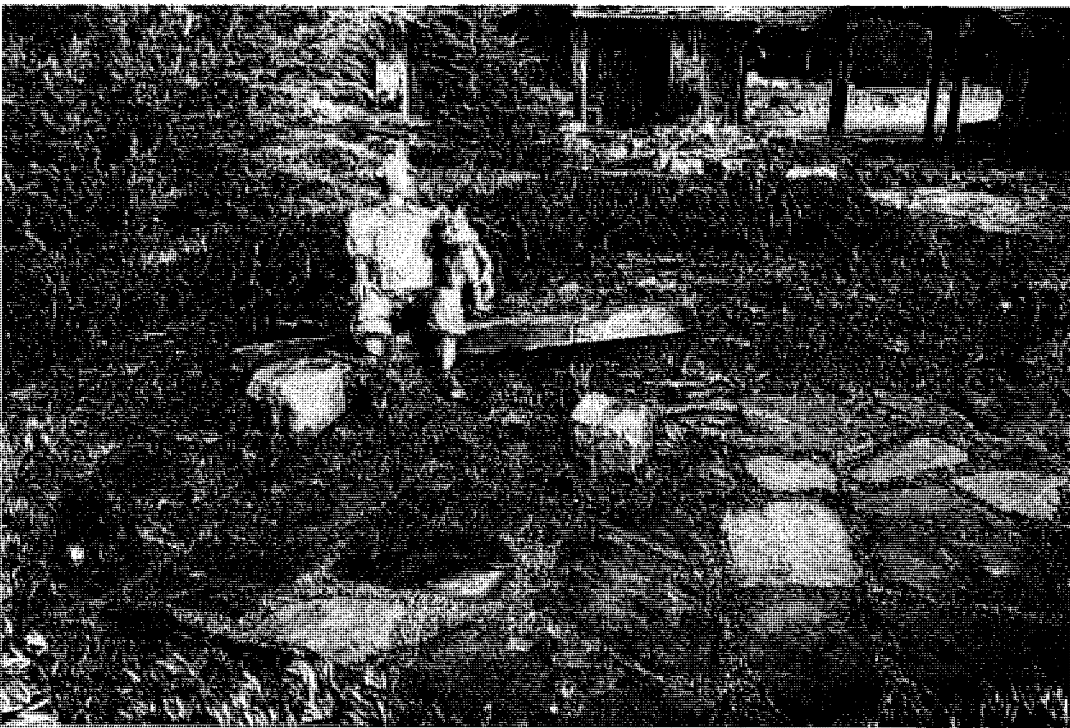
January 2008 overtopping evidence on west side of home, where ice plant and other debris has been carried landward to the back of the Read home by wave runoff.
