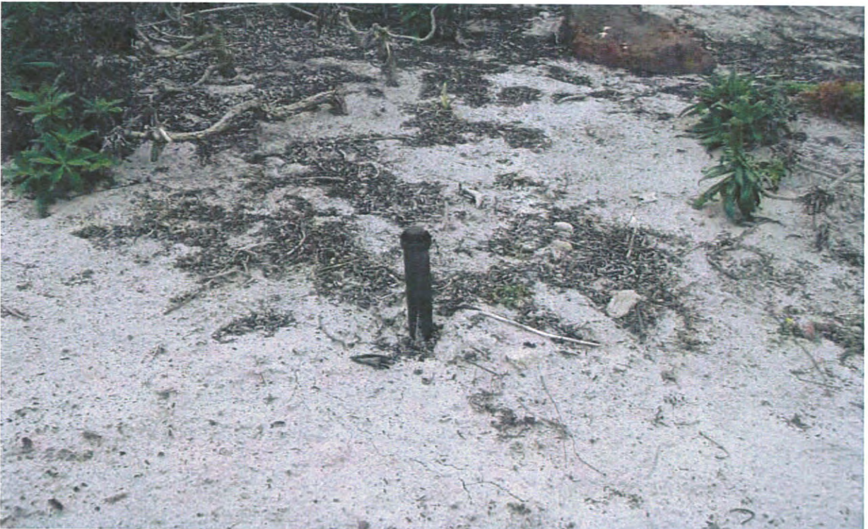
Sprinkler head at edge of mixed landscape area
