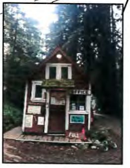
Overhead Attached Down-light at Camping Office
