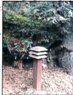
Low Level Bollard Down-lighting
