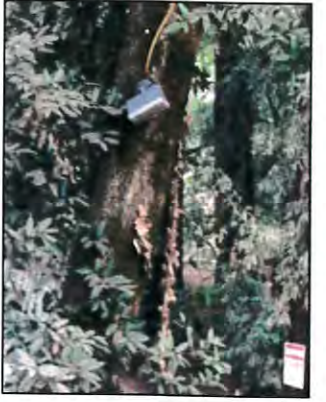
Overhead Pole Lights
