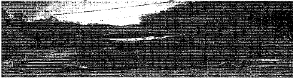
Figure 2: Photo of Damaged Structure
