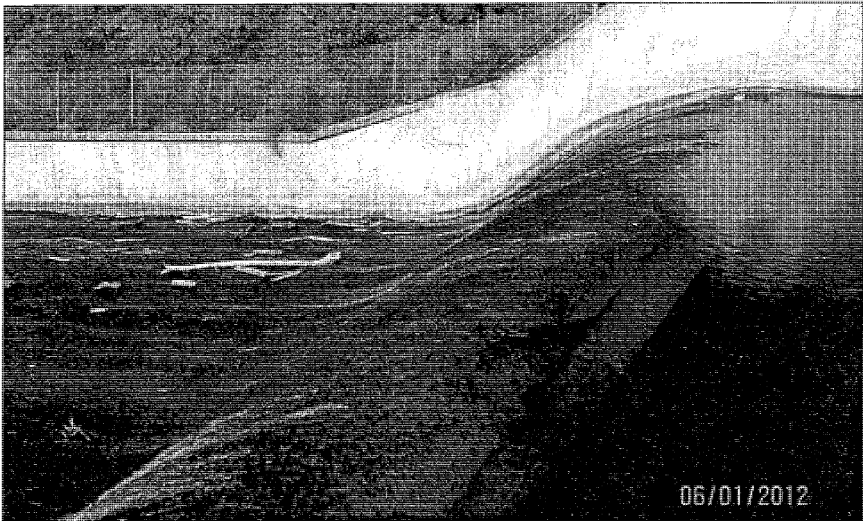
Lip of upper spillway, photographed June 1, 2012. Note flow depth less than 3" and debris obstructions.
