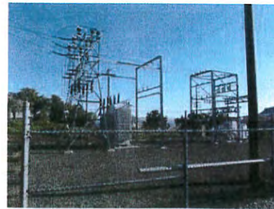
Photo 8. A typical substation with step-up transformer
