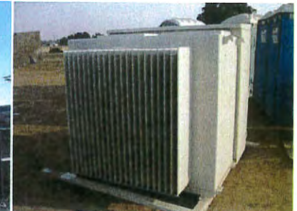
Photo 9. A step-up transformer
