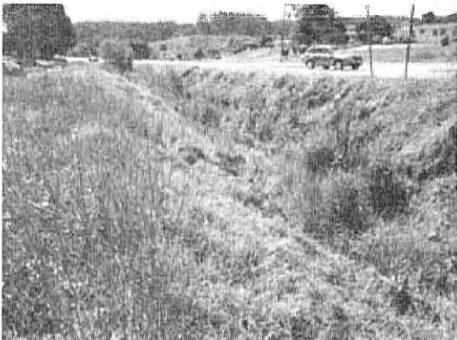
② Unlined portion of drainage channel, east from intersection of Hall Road and Las Lomas Drive
