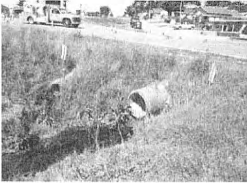
① Outlet of culverts under Las Lomas Drive to drainage channel along Hall Road
