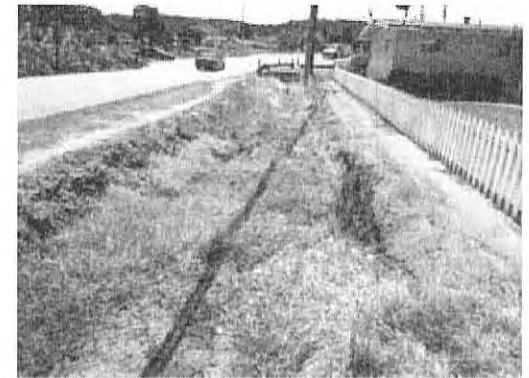
④ Unlined drainage ditch north of intersection of Las Lomas Drive and Hall Road, prior to entering culvert to drainage channel
